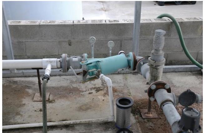
Figure 4. Filter, gauges, and air relief valve. Note flow meter in foreground.
