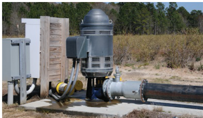
Figure 3. Turbine pump assembly with electrical motor.
